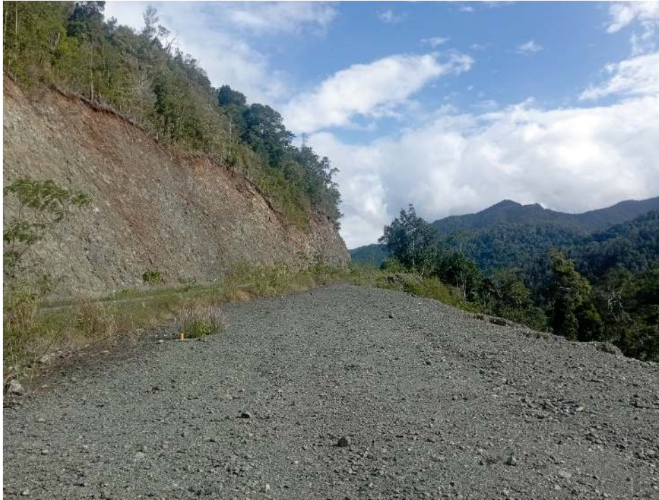
Figure 2 Road-cut slope excavated through highly weathered serpentinite mélange, showing steep slope geometry, intense weathering, and fractured rock mass conditions.
